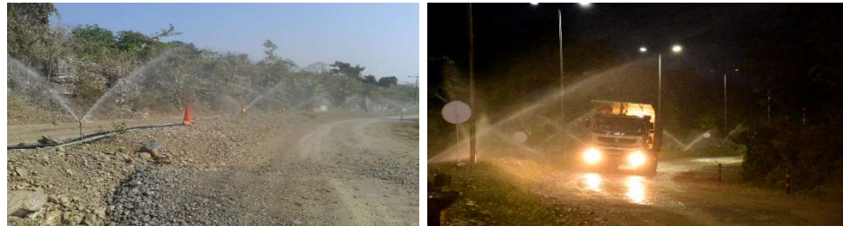
Water Sprinklers fixed along the median of Haul Road.
