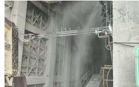
Water Fogger at Dump Hopper
