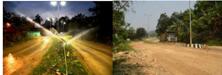
Automatic Water Sprinklers fixed along the median of Haul Road.
